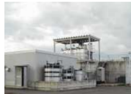
Waste Water Treatment Facilities
