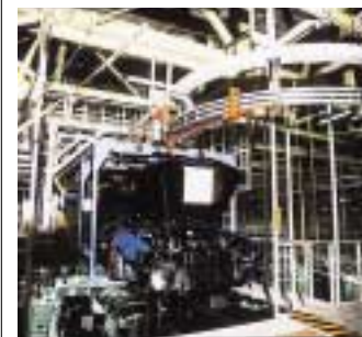
ES Monorail System with the Non-contact Power Supply System
