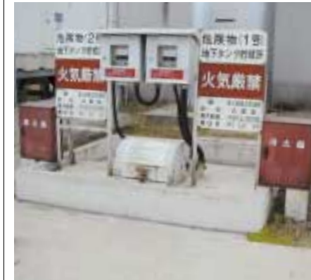
Oil trapping fence
