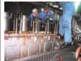
Checking the Cogeneration System
