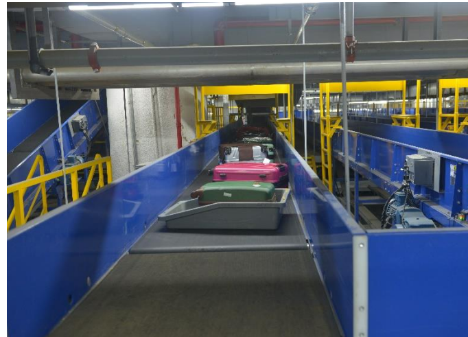
Baggage handling systems
