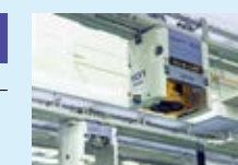
Cleanroom transport systems for semiconductor factory
