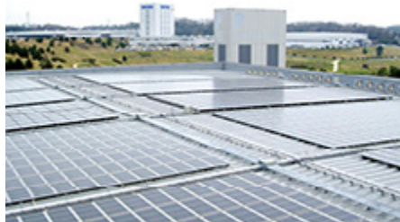
Solar modules installed on the rooftop
