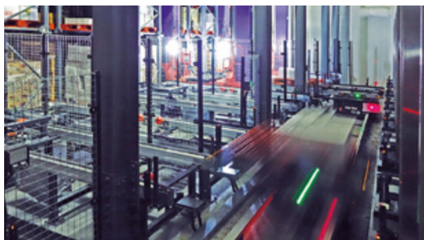
Automated warehouse with earthquake resistant measures
