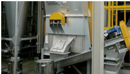
Sludge recycling facility
