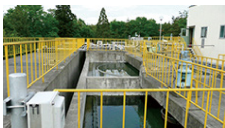
Effluent treatment facilities
