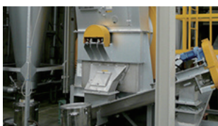
Sludge recycling facility
