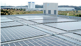
Solar modules installed on the rooftop
