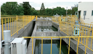
Effluent treatment facilities
