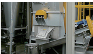
Sludge recycling facility
