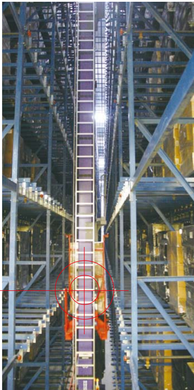
All 12 stacker cranes store pallets double deep
