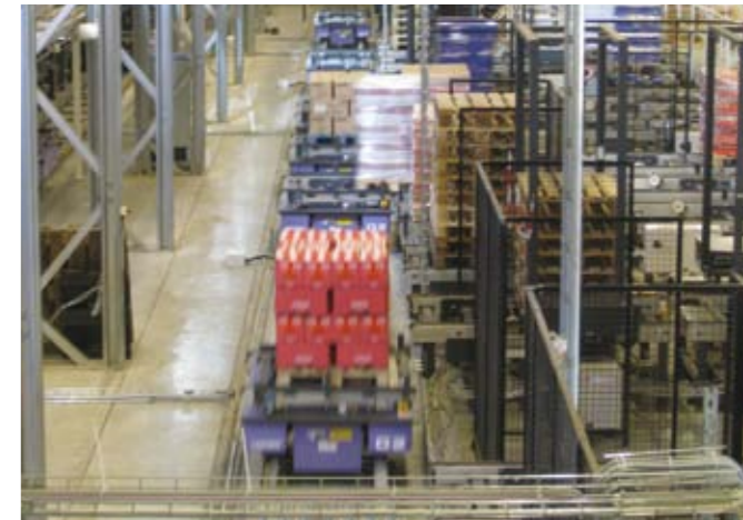
29 high-speed rail-guided sorting transfer vehicles on a loop track transport incoming shipments
