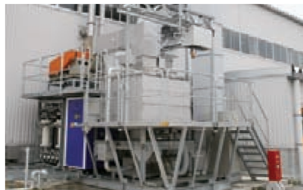
VOC remover installed at the Shiga Works
