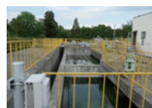
Effluent treatment facilities at the Shiga Works
