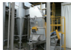
Sludge recycling facility
