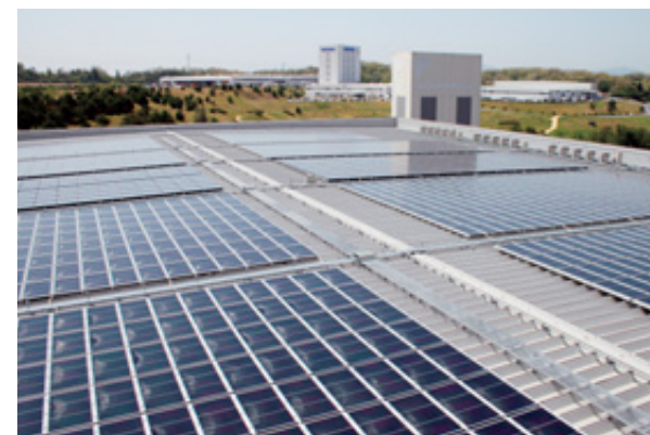
The roof-mounted solar modules are 70 meters long and 60 meters wide.
