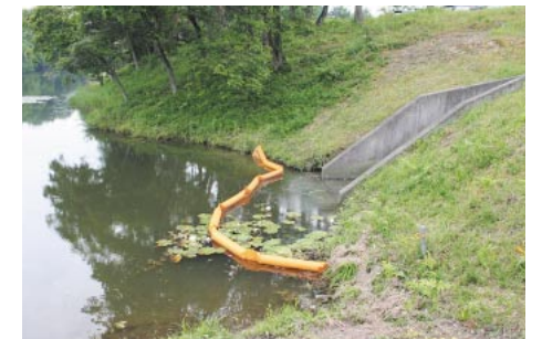
Oil barrier at a fire prevention pond at the Shiga Works
