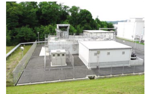
Drainage treatment facilities at the Shiga Works
