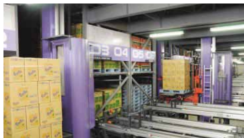
The automated warehouse with nine stacker cranes and 33,408 pallets
