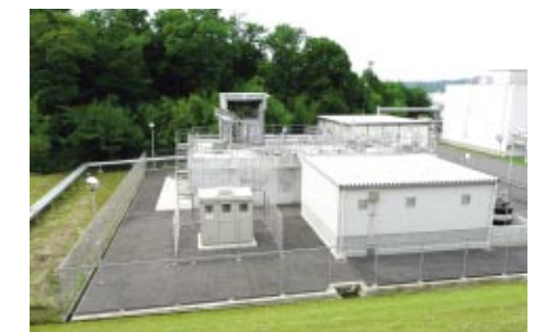
Drainage treatment facilities at the Shiga Works
