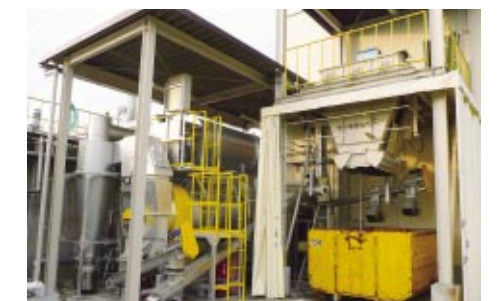
Sludge recycling facilities
