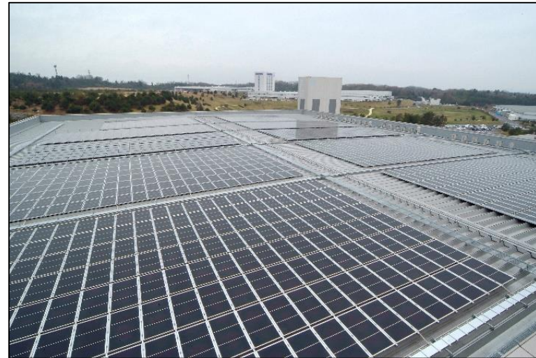
Solar panels installed within Daifuku's Shiga Works
