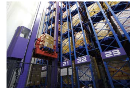
Automated freezer warehouse system delivered to a food product manufacturer in Thailand
