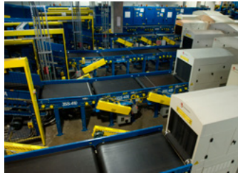
Baggage Handling Systems
