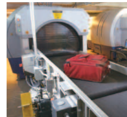
Airport baggage handling system
