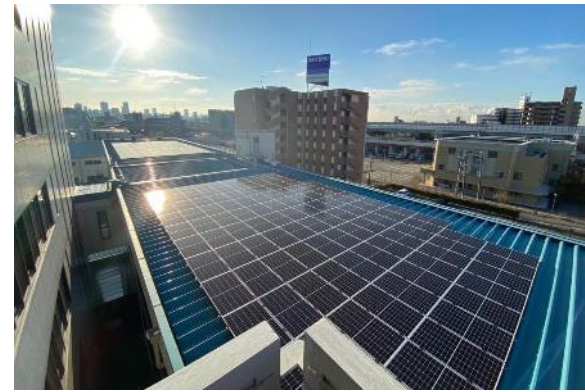
Contec Co., Ltd. Headquarters introduced a rooftop photovoltaic system in 2022.
